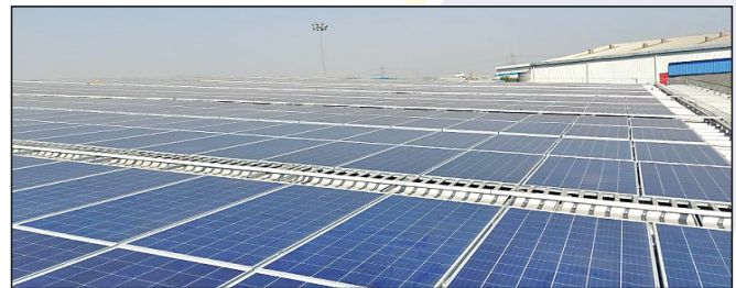
1 MW Solar project at Yeola, Nashik
