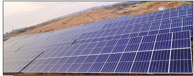
600 kW ground mounted project at Jalgaon
