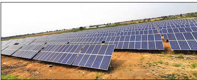
1 MW Solar Power Plant at Akola
