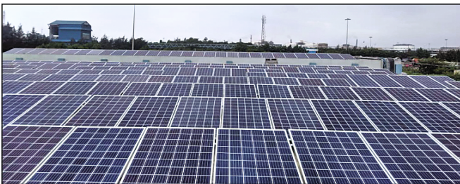
2 MW Solar Power Plant at Bhandara
